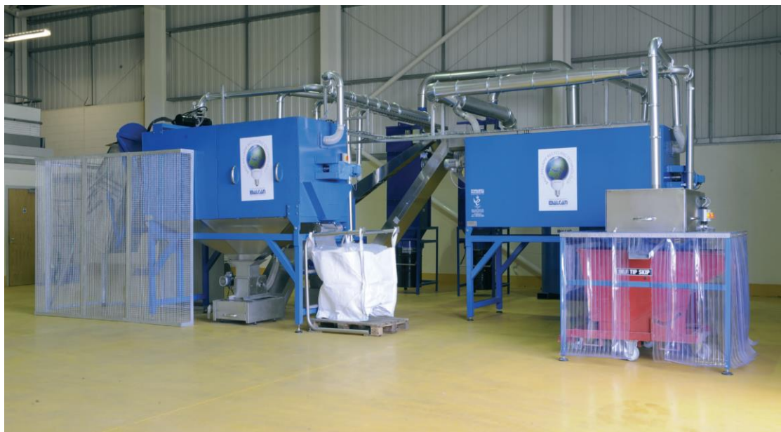
Figure2 BALCAN M 6000-U.K recycling plant operated in BIS RecyclingCenter, Omoljica, Serbia (Q = 5 mil. Lamps / year )
